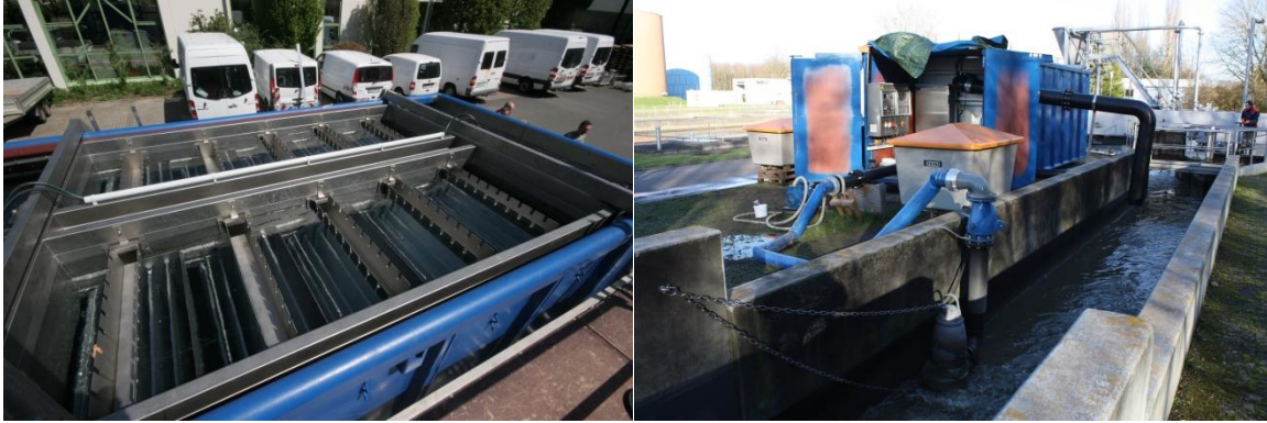
Figure 4: Upflow lamella container. Left: Top view with lamella modules and overflow system. Right: Container in place. In the foreground the feeding pump in the inlet flume of a treatment plant and one of the 1000 L samplers
